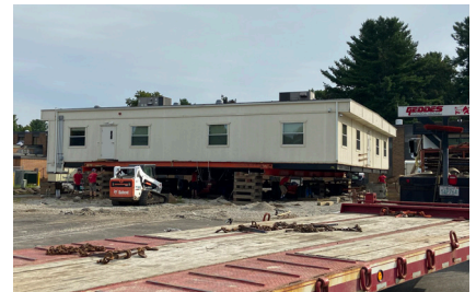
Above: Portable relocation.
